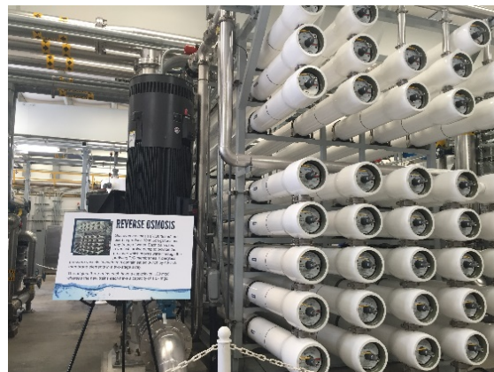
Reynolds Desalination Facility
