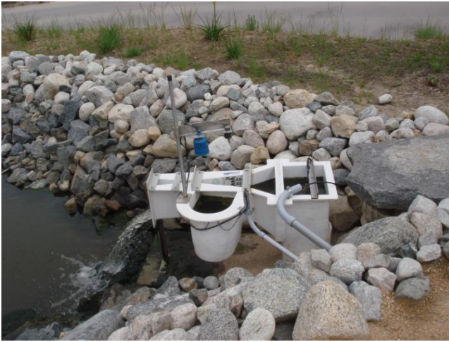
Water quality monitoring data collection site at the Biofiltration Wetlands (San Diego Zoo Safari Park), partially funded through the IRWM Program.
