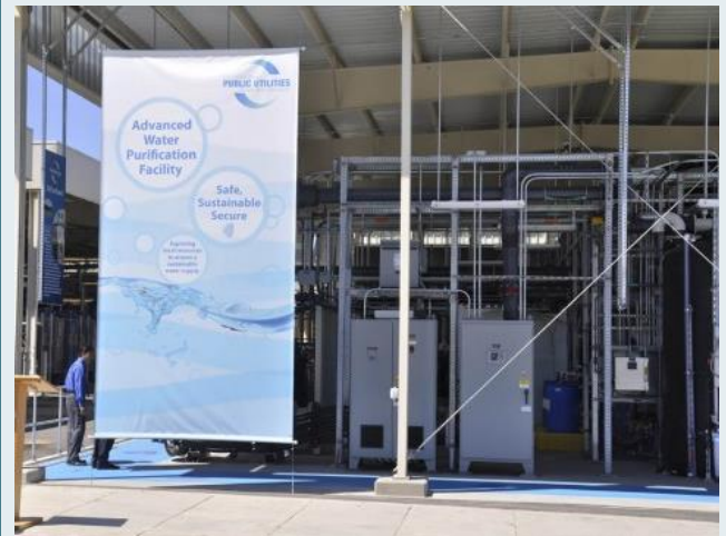
The City of San Diego Advanced Water Purification Facility is conducting pilot testing for indirect potable reuse.
