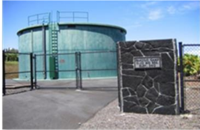
Aging storage tanks can lead to contamination of rural water supplies.
