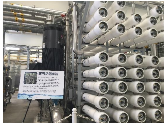
Reynolds Desalination Facility
