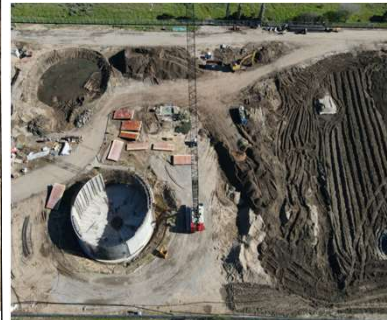
East County AWP Project, Site Preparation and Concrete Work – SHF and Digesters
