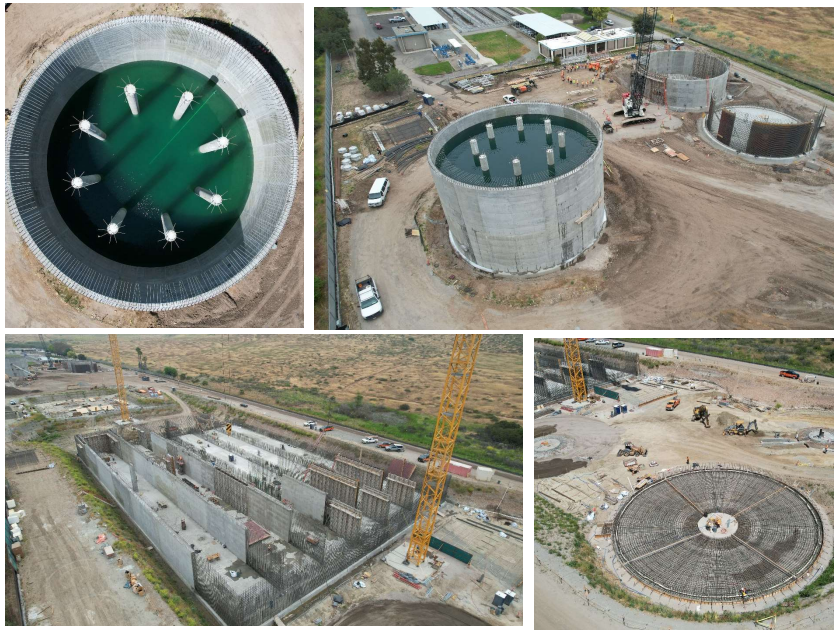
New treatment facility construction update: Shown at the pictures are three digesters, aeration basins, and secondary clarifiers
